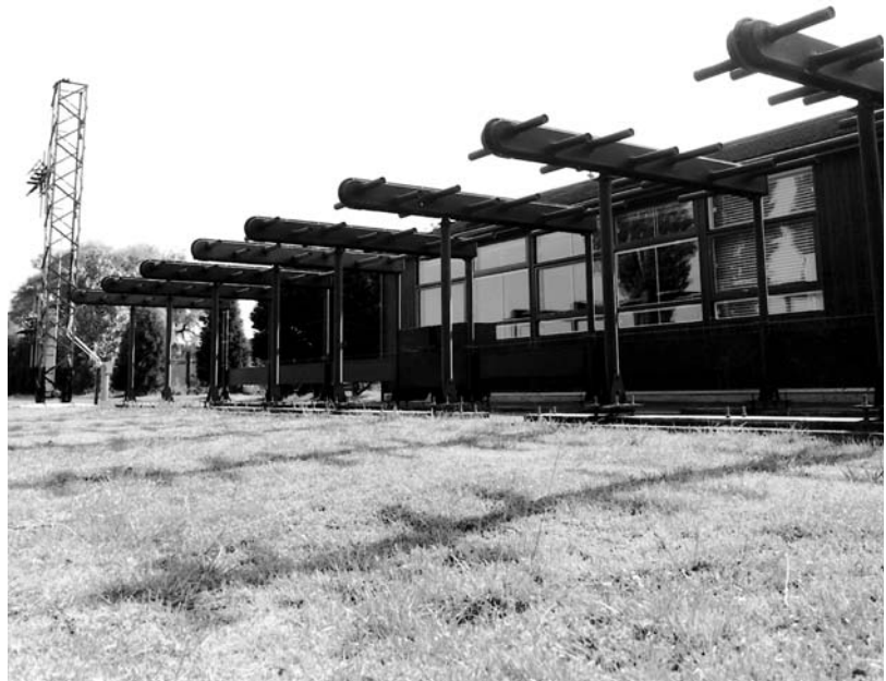
Fig 4-7: The ILS localiser aerial (note the photograph shows a technicians training setup. There would be no office block at a real site)
